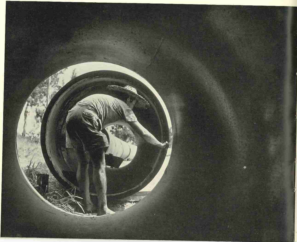
New pipe-lines being built to receive water from Shumchun Reservoir on mainland
