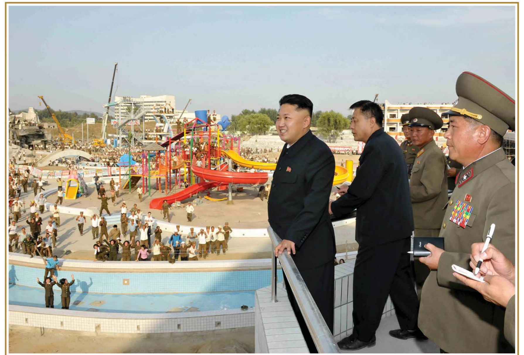
Supreme Leader Kim Jong Un visiting the construction site of the Munsu Water Park [September Juche 102 (2013)]
