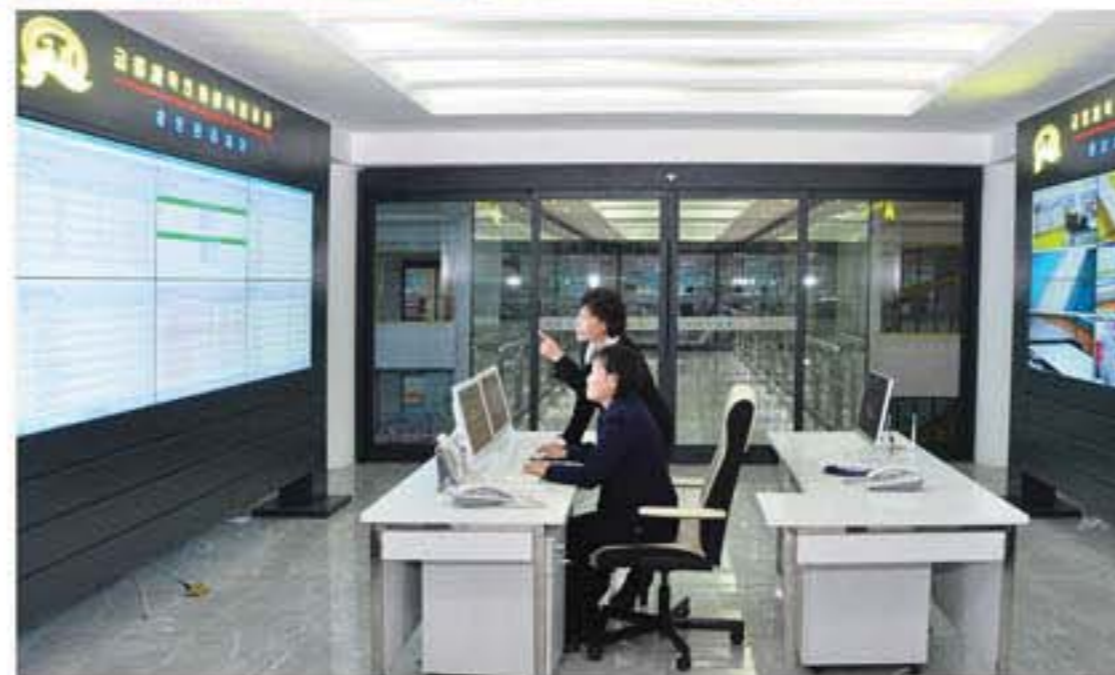
General control room
