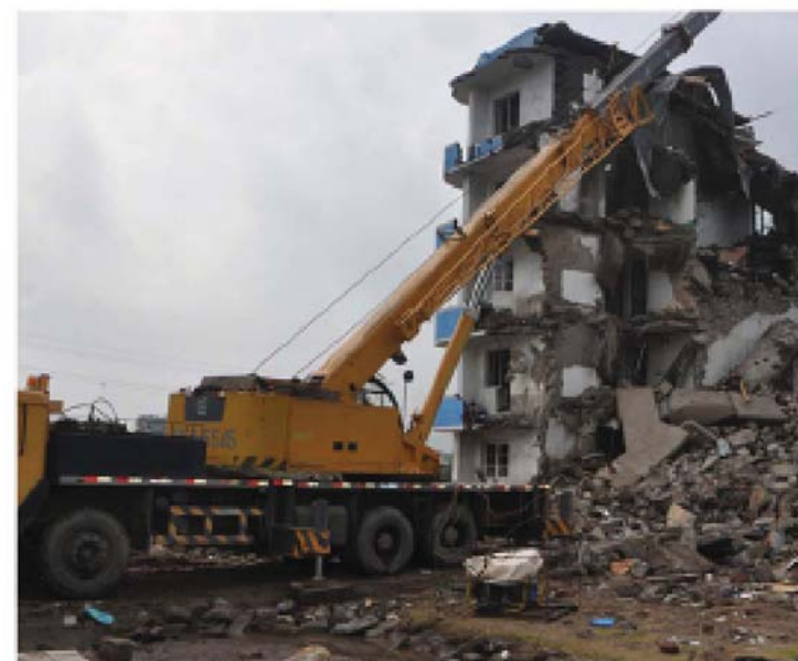
Many dwelling houses and public buildings in some areas of Rason were collapsed by the unusually heavy rain in August
