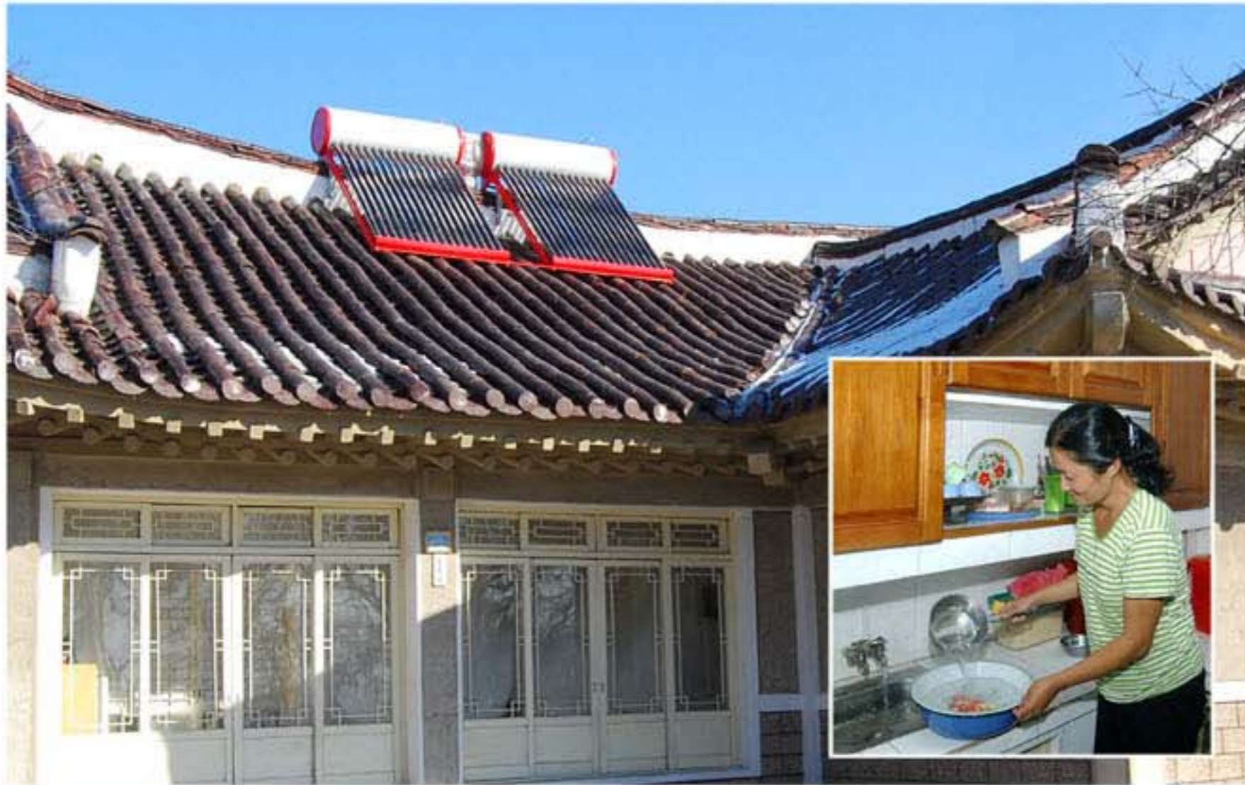
Solar water heaters are installed in the houses
