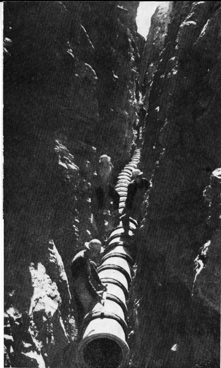
Water pipes cutting through mountains.
