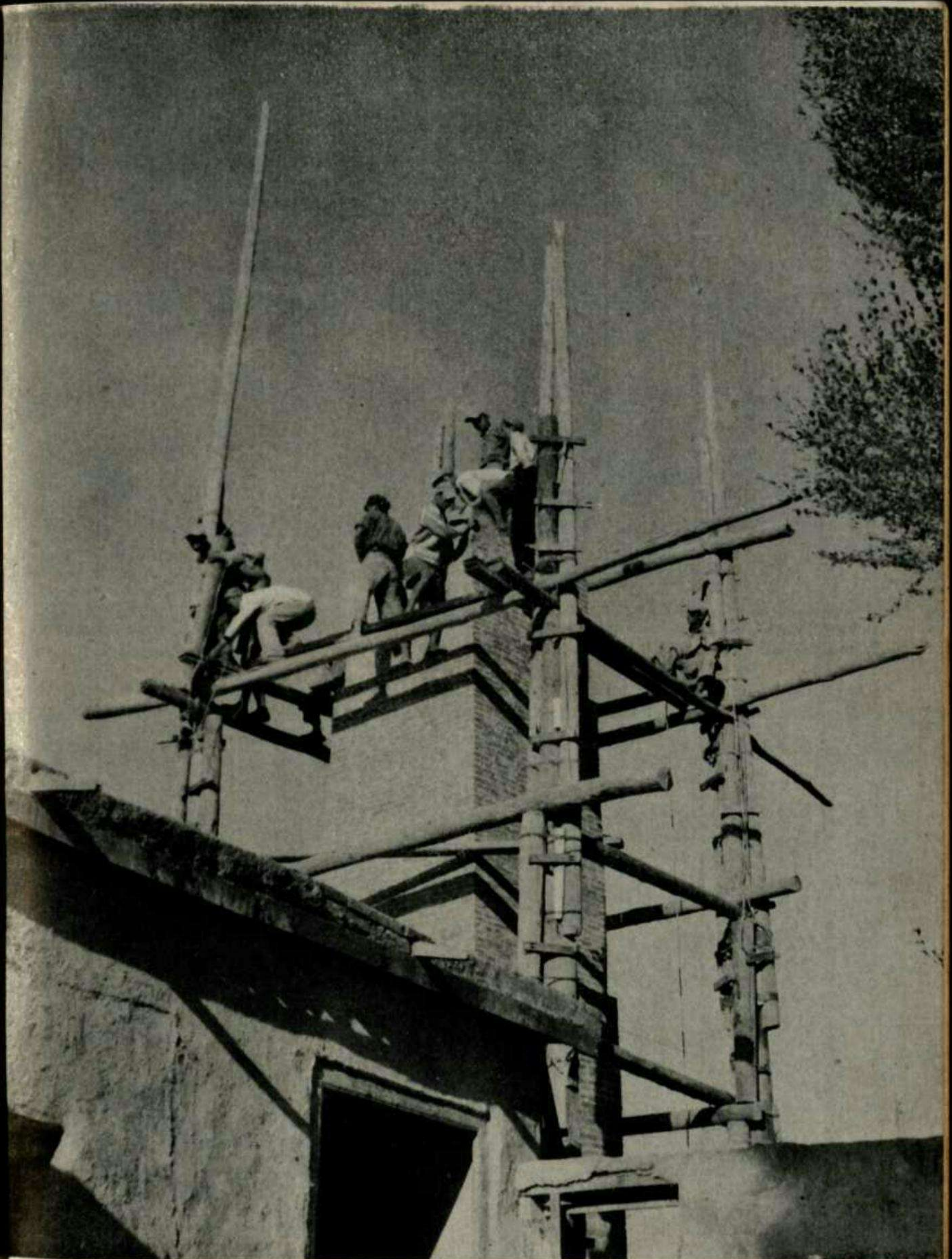
Joint Effort: Boys of Bailie School ceramics section help textile students put up new chimney for dyeing and wool washing plant.
