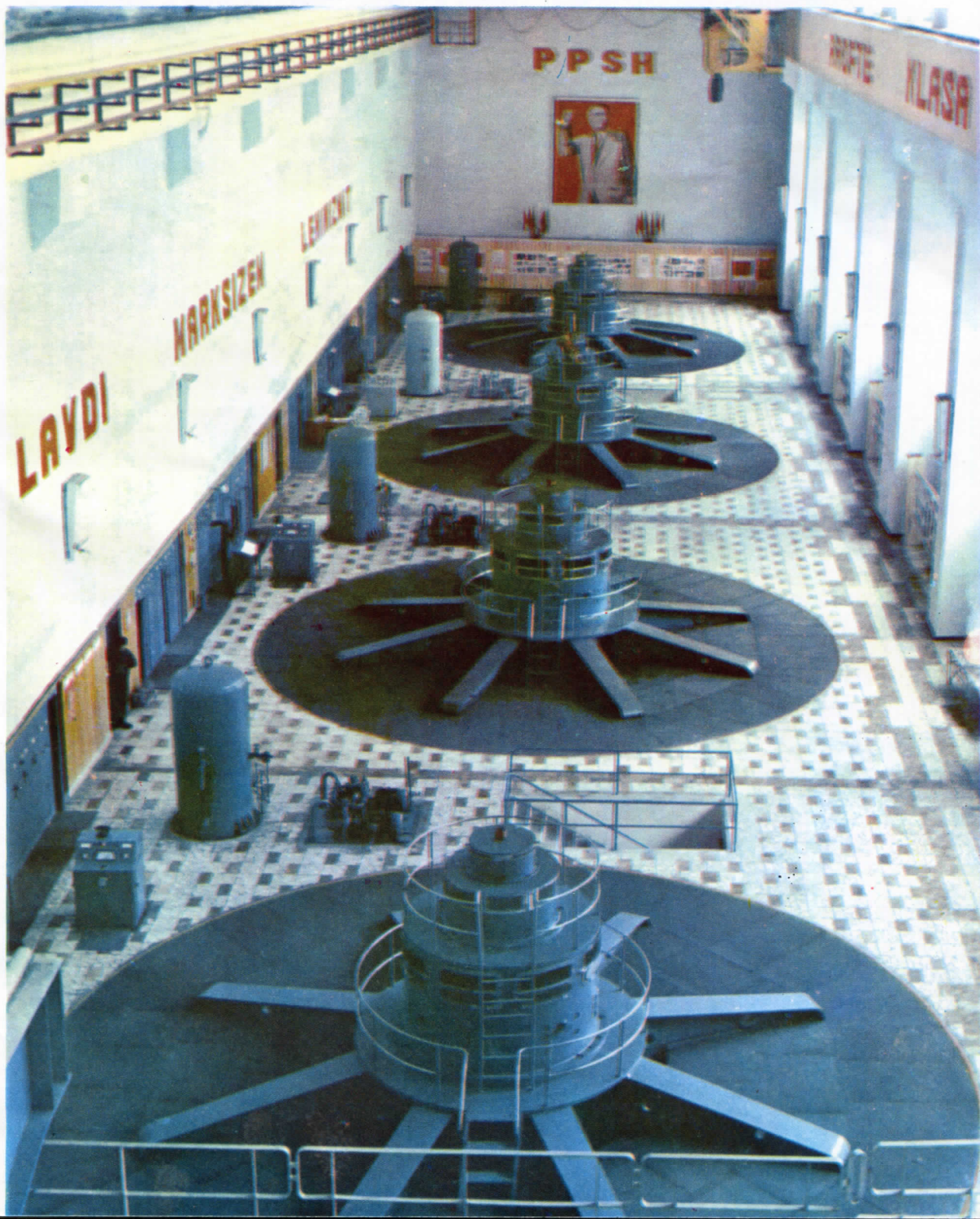
View of the turbine section of the «LIGHT OF THE PARTY» hydro-power station at Fierza.
